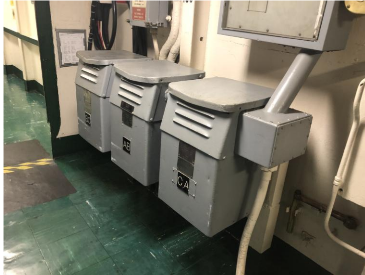
Figure 1: Transformer bank onboard USS Midway CV-41 (photo by Norbert Doerry)
